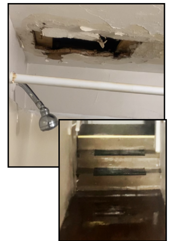
Water damage at an Elmwood Realty property. Photos courtesy of Plaintiff Jordan Towns.
